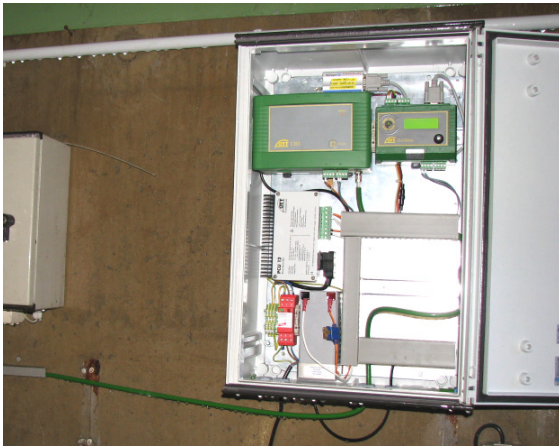
Innerste Dam control way – Water storage level measurement OTT CBS 30 m , OTT DuoSens , GPRS data transmission
